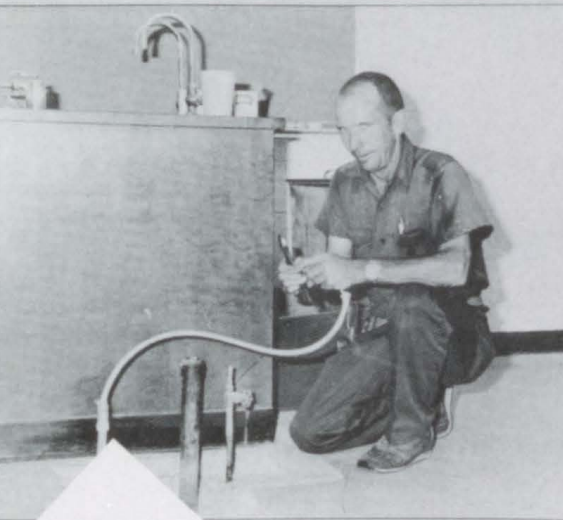
DONNIE HOLCOMB works on plumbing being installed in the new high school lab facilities. The lab should be completed Oct. 1 and carries a price tag of approximately $7,200. (Photo by George Bridges)
